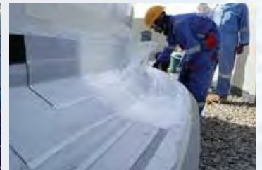
Tank Base Protection
